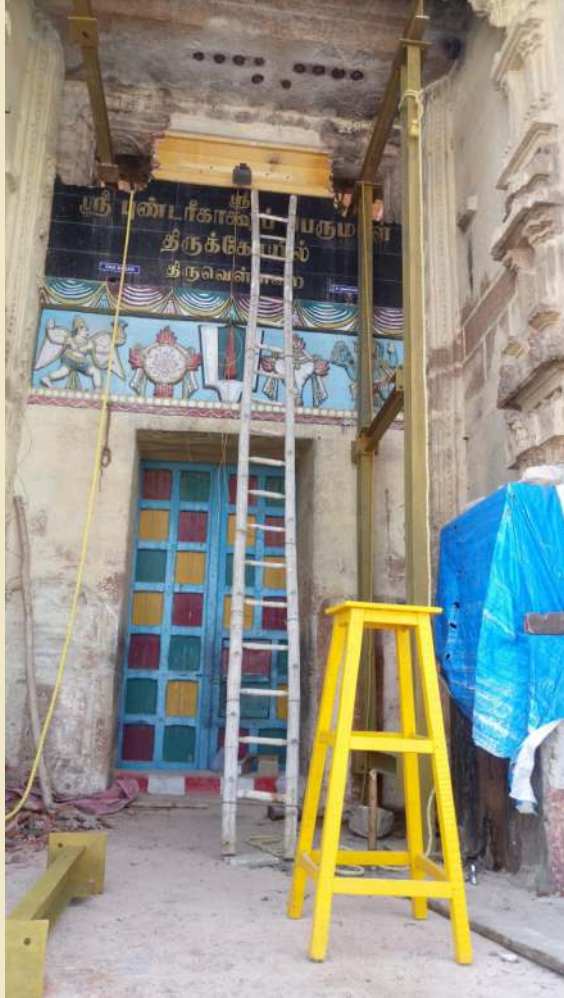
This was the main RajaGopuram entrance, 6 feet width x 10 feet height that was in use since 1965 to March 2019
